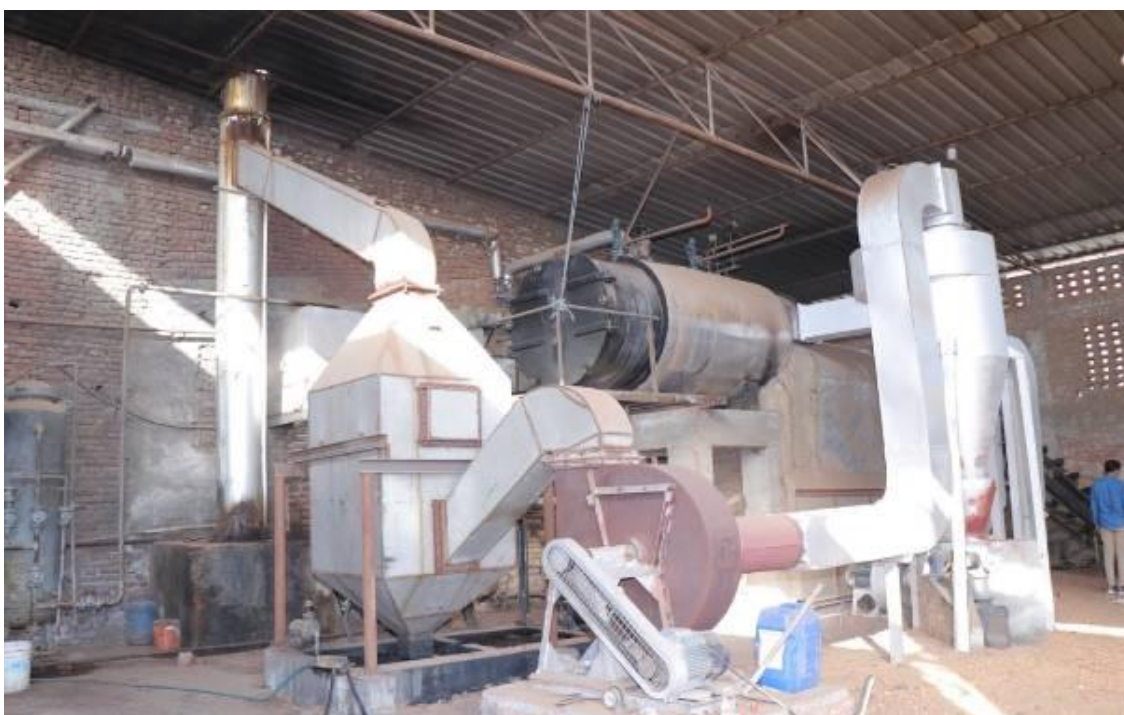
Figure 23: Air Pollution Control System in Shakun Handifab Pvt. Ltd. Partapur, Meerut city
